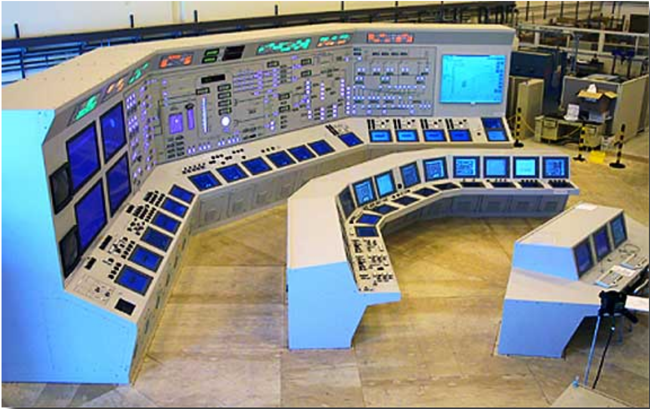
Figure 2-5. ABWR (Lungmen) Main Control Room Panels
